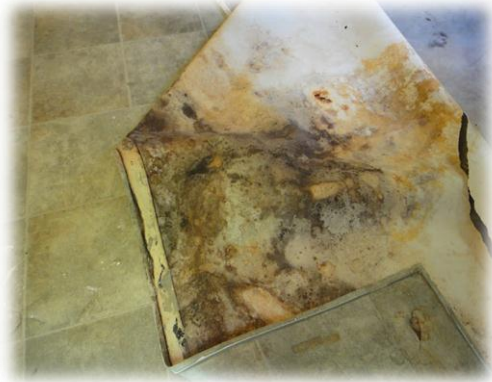
Figure 7: Defect on carpet caused by condensation on concrete slab
