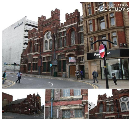
Case Study 5: Former Salvation Army Citadel Building, Cross Burgess Street, Sheffield, South Yorkshire.
