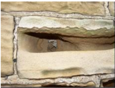
Figure 3: Example of cavernous weathering, southern elevation Norwood Piggeries
